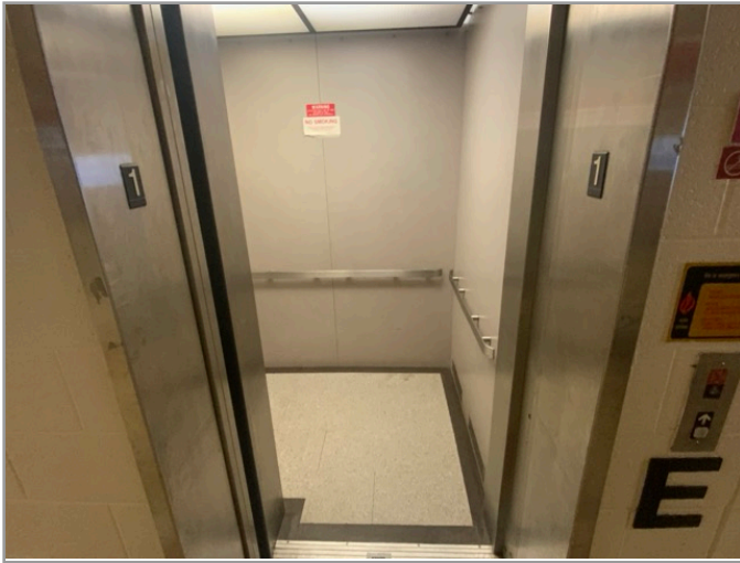
LOBBY LOOKING AT CAB
