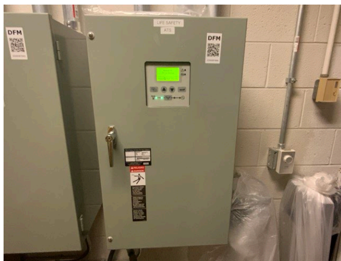
24 - AUTOMATIC TRANSFER SWITCH
