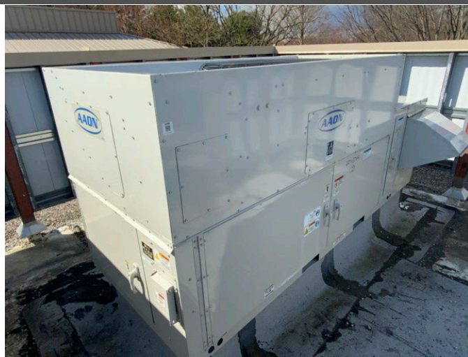
20 - ROOFTOP PACKAGED UNIT
