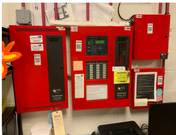
22 - FIRE ALARM DEVICES
