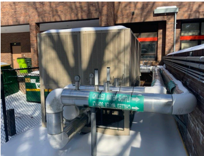
15 - AIR COOLED CHILLER
