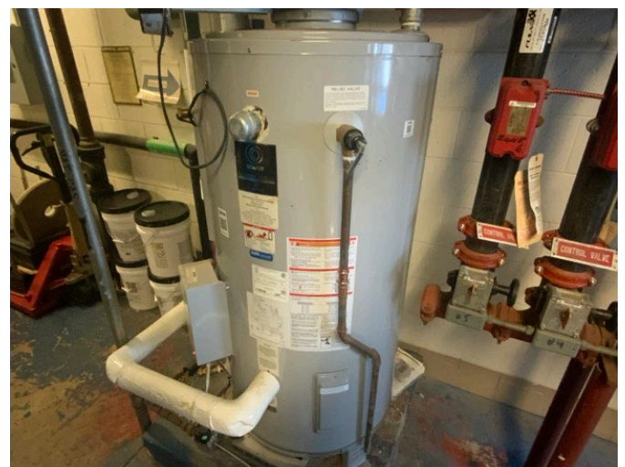
12 - GAS FIRE WATER HEATER
